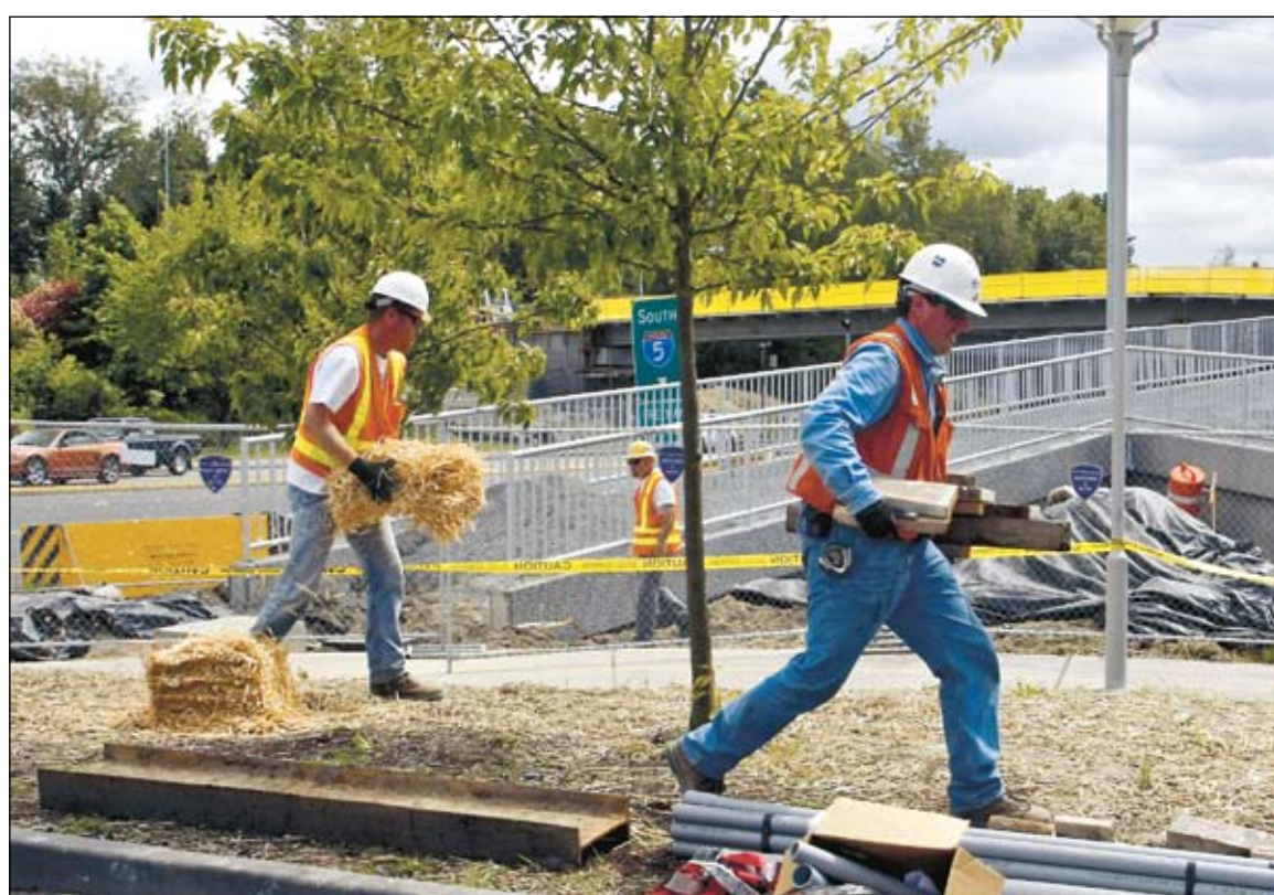
Construction workers Matt VanLier (left) of Allied Construction Associates in Everett and foreman Rich Bovard of Seahurst Electric move materials where a pedestrian bridge over 44th Avenue West in Lynnwood is being built.
